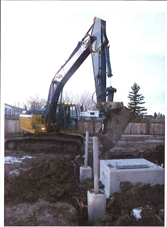
Electrical Pedestal for Fortis
