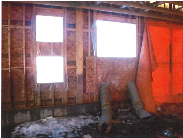
Temporary Heat Supply
